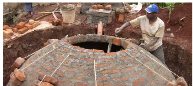
One of the first biogas units just before completion. At the moment more than a dozen specialised masons are doing the construction work of the installations.
